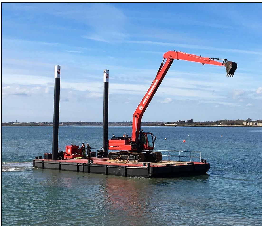
Plate 11.16 Example of Spud-can Barge with long-reach excavator to be used in the construction of the works.
